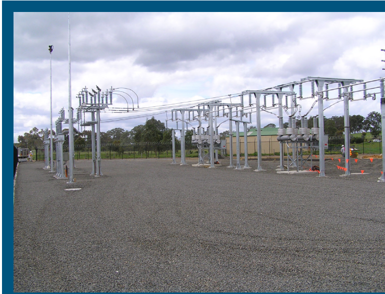
66kV Bus installation at the Doreen Zone Substation
