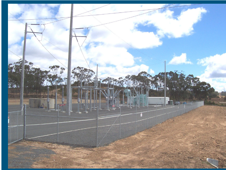
Fosterville 220kV Terminal Station
